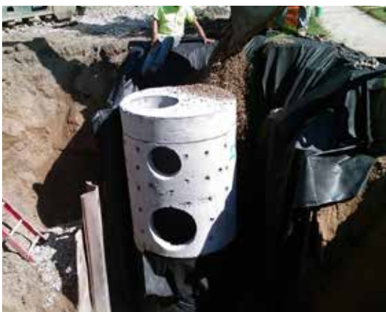
Figure 25. The City has installed a number of infiltration basins around town to capture stormwater near where it falls to help it slowly seep back into the ground. Photo: Grand Rapids Environmental Services Department
