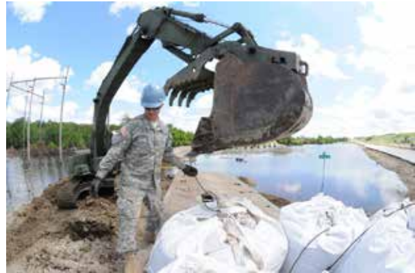
Figure 21. Horizontal Engineering Company works with the Minnesota Army National Guard to repair a levee. Photo: Sgt. First Class Daniel Ewer, U.S. Army
