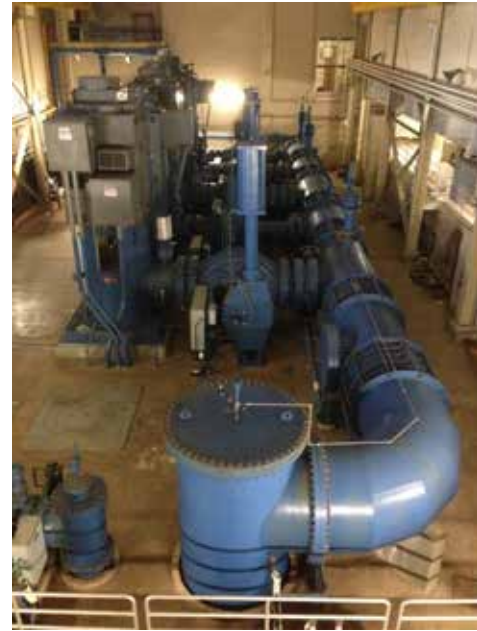
Figure 32. Massive pumps move treated, potable water from the water filtration plant in West Olive to Grand Rapids. The energy/water nexus goes both ways; saving water saves energy.
